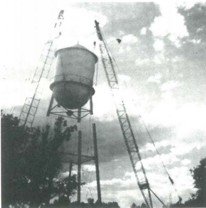
The Mills water tower being taken down and moved to Wardwell in 1975. Courtesy Larry Edwards.
